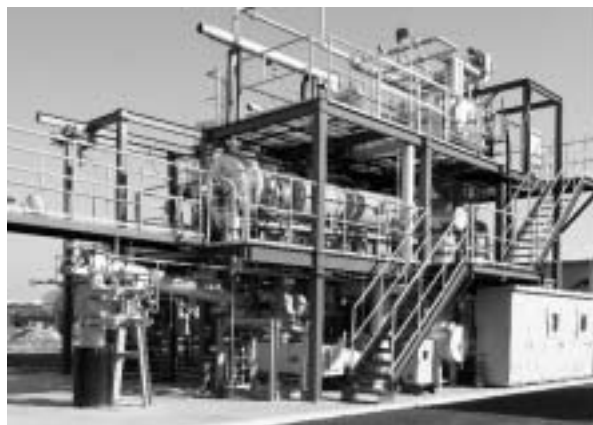
図7 実証実験設備 Fig.7 View of pilot plant.
