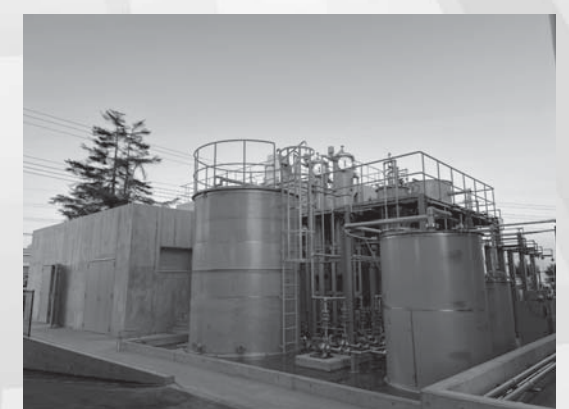
図10 排水処理設備 Fig.10 Wastewater treatment facility.
