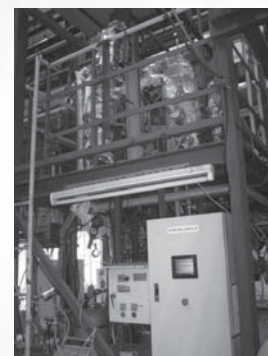
図4 TSA 型溶剤回収装置 Fig.4 Temperature Swing Adsorption
