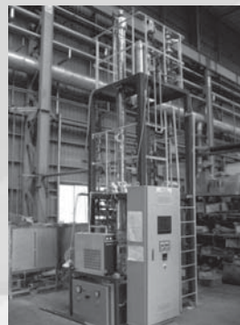
図3 触媒湿式酸化装置 Fig.3Catalytic Wet Air Oxidation Wastewater Treatment System
