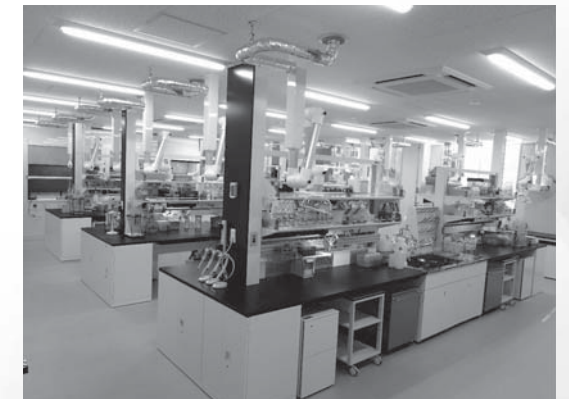
図9 事務所棟 分析室 Fig.9 Chemical analysis room in office building.
