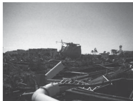
図1 震災後の被害状況（最初沈殿池周り） Fig.1 Damage around the primary sedimentation tank after the Great East Japan Earthquake
