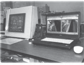
図7 汚泥処理監視室内の遠隔操作用TPと映像用PC Fig.7 Touch panel for remote operating and computer for monitoring
