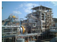
Solid waste treatment facility
