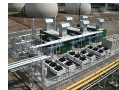
Digestion gas power generation business
