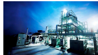
Dehydration and drying system
