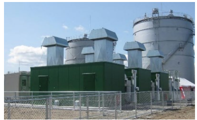
Shinjiko East Power Station
