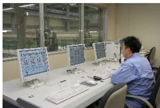
Operations room at sewage treatment plant
